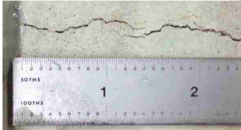
Figure 3.17: Cracking along the surface of the specimens containing uncoated rebar.
